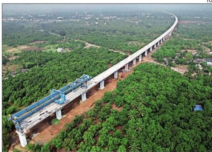
HSR stations at Vapi, Bilimora, Surat, Bharuch, Anand, Vadodara, Ahmedabad and Sabarmati in Gujarat are at various stages of construction
